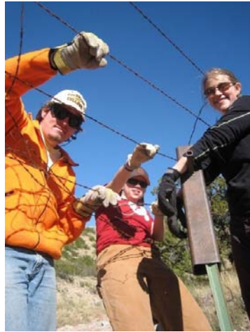
Students work together to repair barbwire fences at Sevilleta National Wildlife refuge in New Mexico
